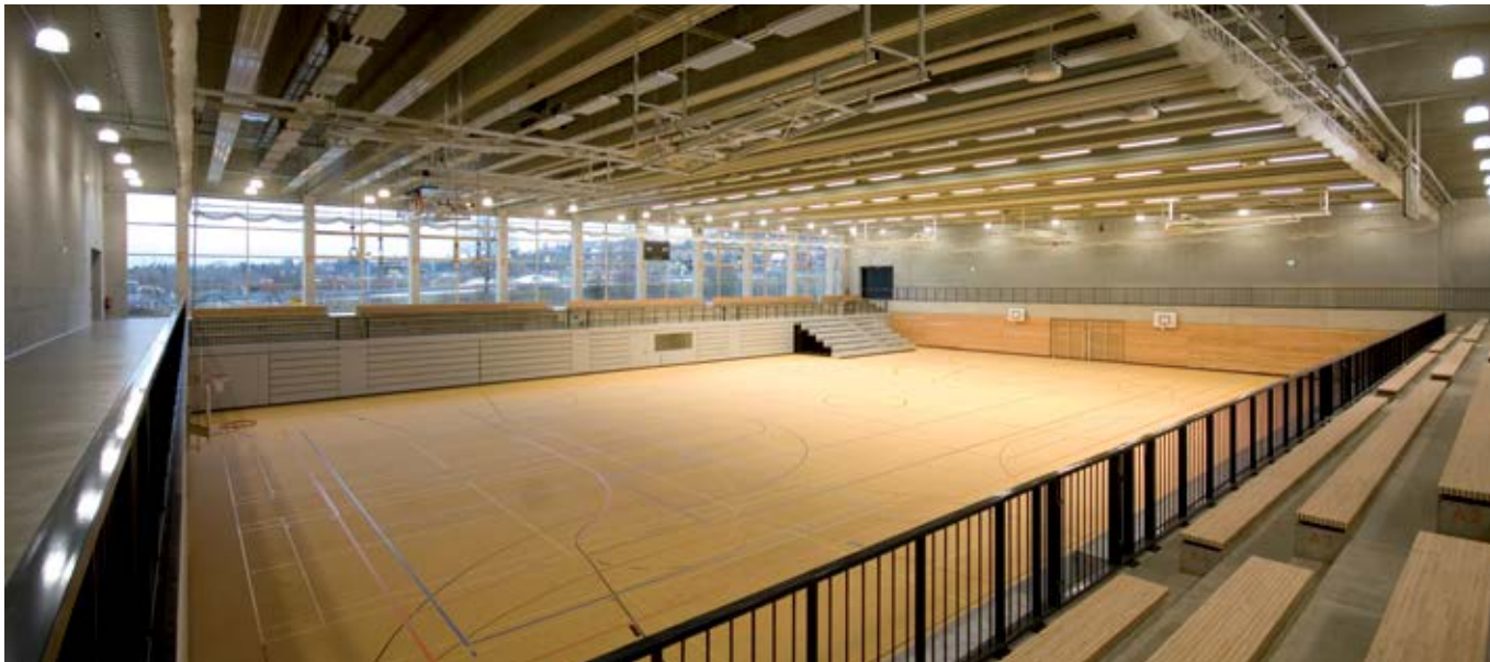
Presence detectors mounted at a height of ten metres also take account of daylight coming through the windows at the front when controlling light.
